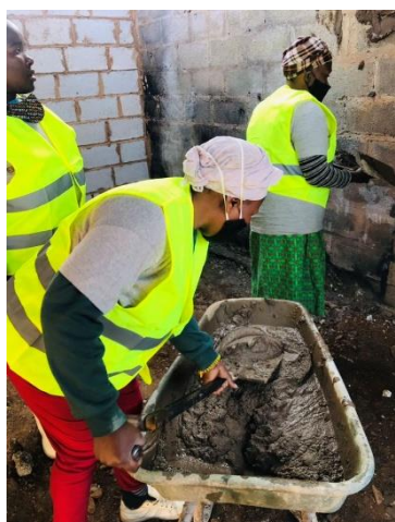
Survivors from the SWITs skills development programme put their building skills to action by building a house for a fire survivor.
